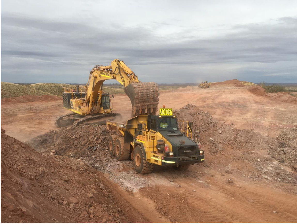
(Figure 2: First load of mineralized conglomerate being loaded into an articulated truck. The flat area in the background is pre-stripped of waste. The D9 bulldozer in the far distance is removing the final waste material.)
