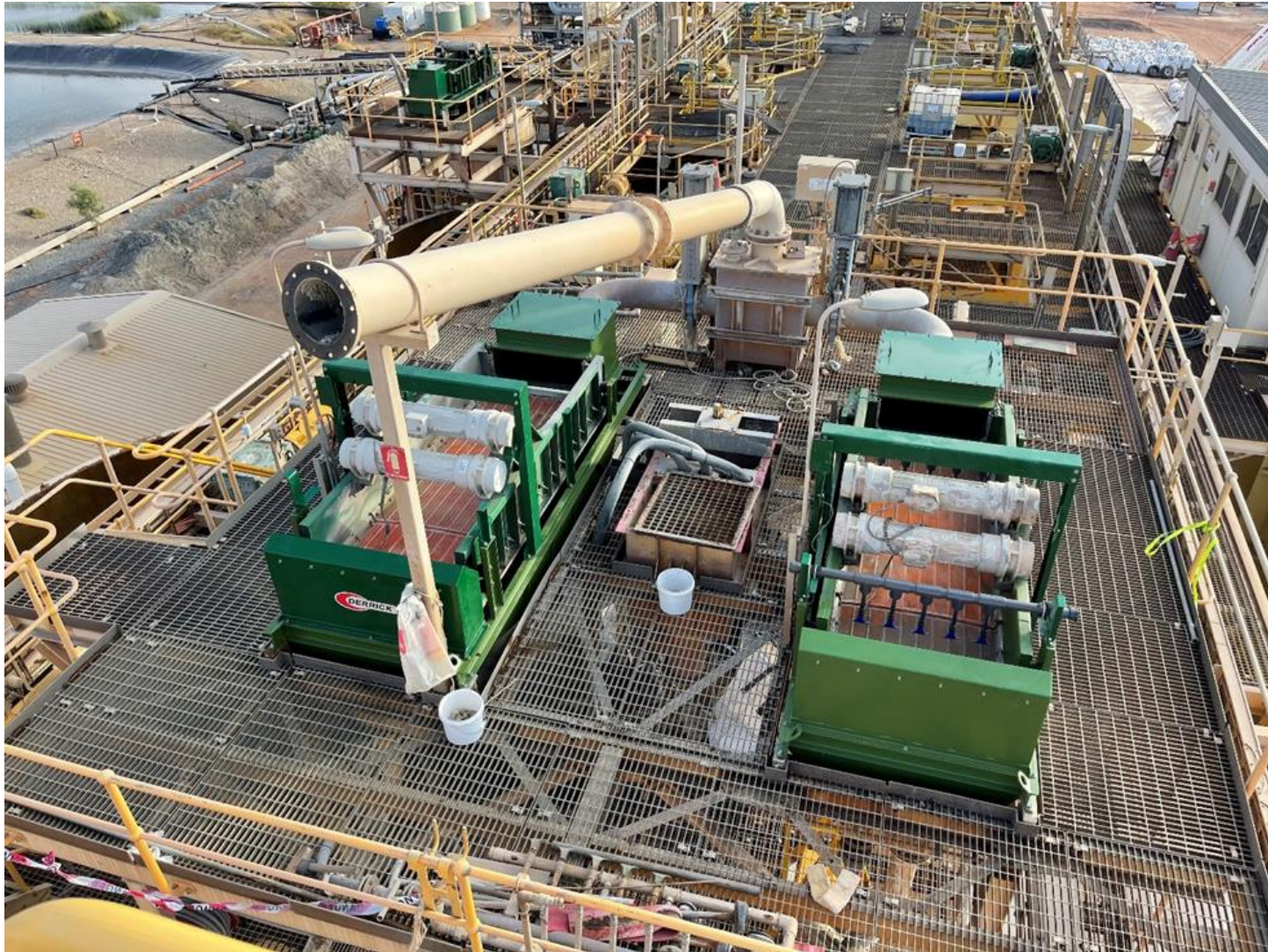
(Figure 3: Fully refurbished and re-installed trash screens on the Golden Eagle Mill.)
