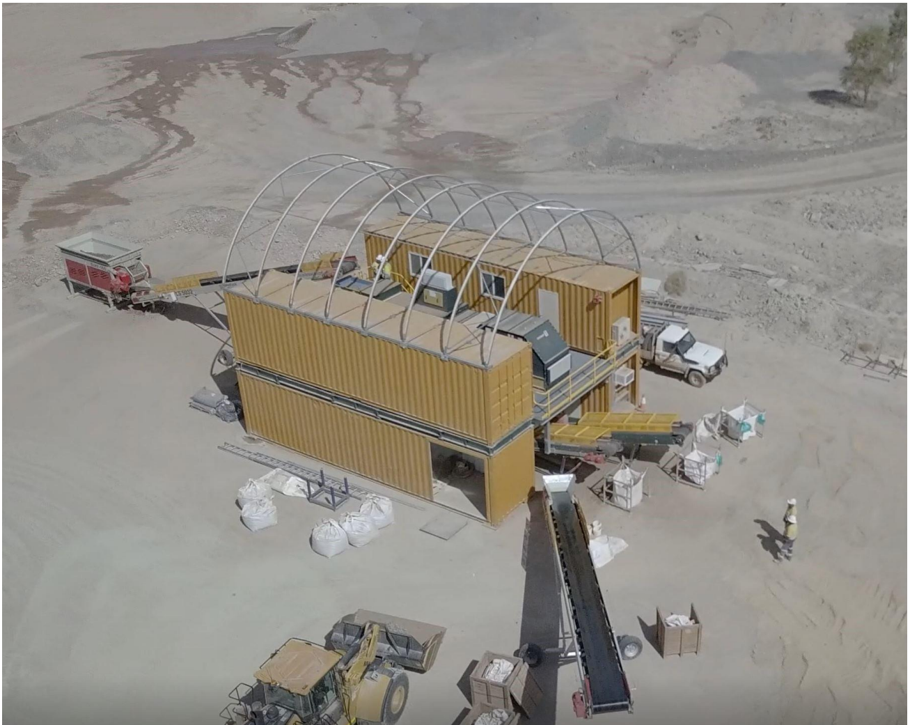
(Figure 1: The Sorter and associated infrastructure undergoing final construction and commissioning at the Nullagine Gold Project.)
