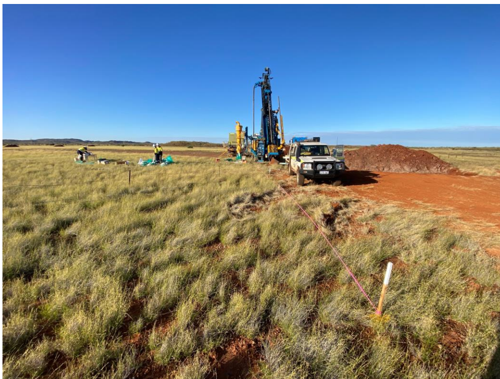
Figure 4: RC drill rig at the Morto Lago Prospect, in the Karratha District.
